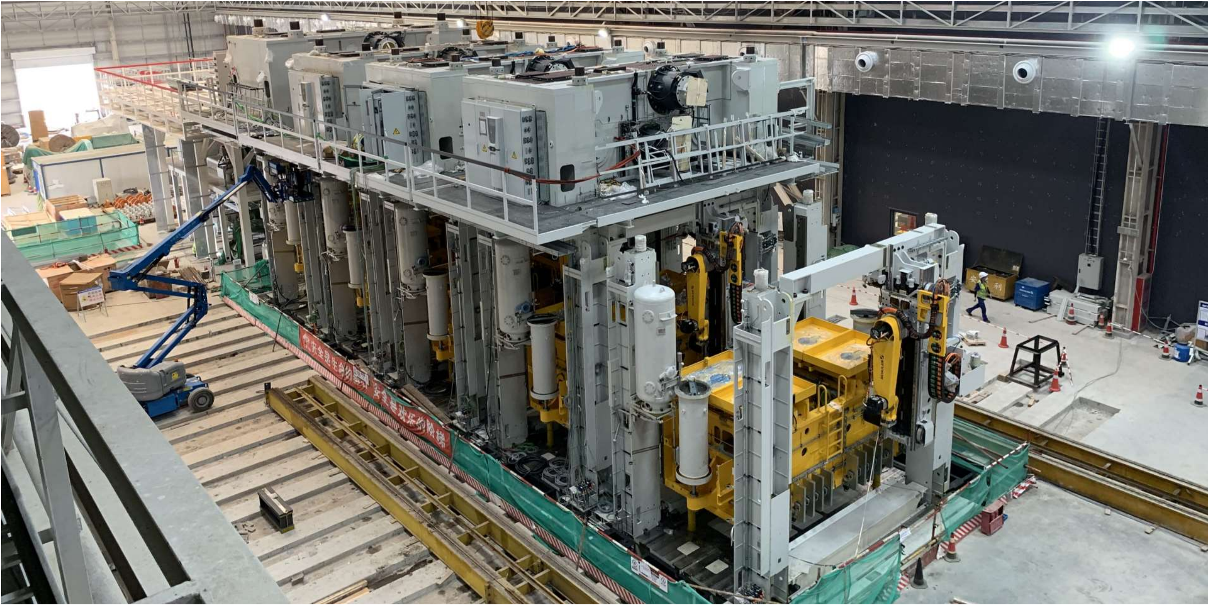
GIGAFACTORY SHANGHAI - MODEL Y FACTORY INTERIOR
