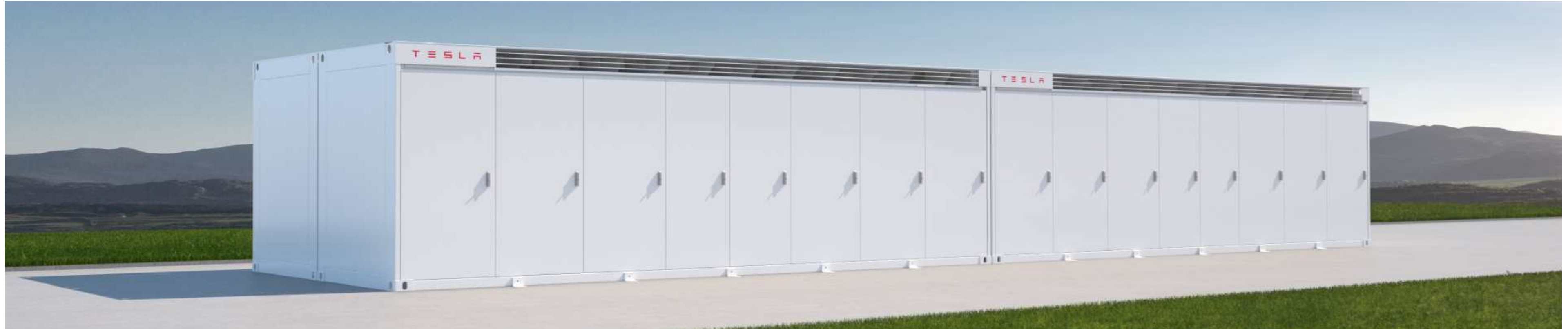
Megapack - 3 MWh battery
